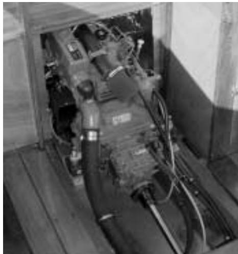
The new MD2030 installed.
